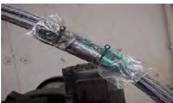
Bottom Deadend and Hardware Tie-Wrapped to Guy Kit
