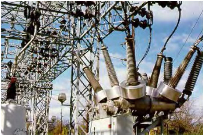
Dead Tank Breakers
